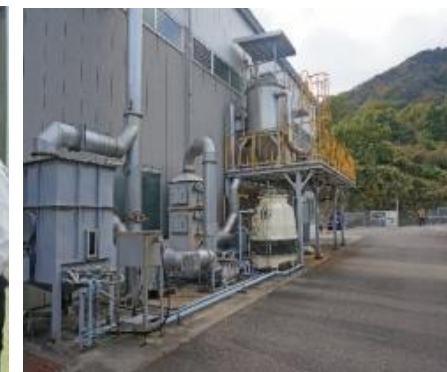
Outdoor exhaust gas and wastewater treatment
